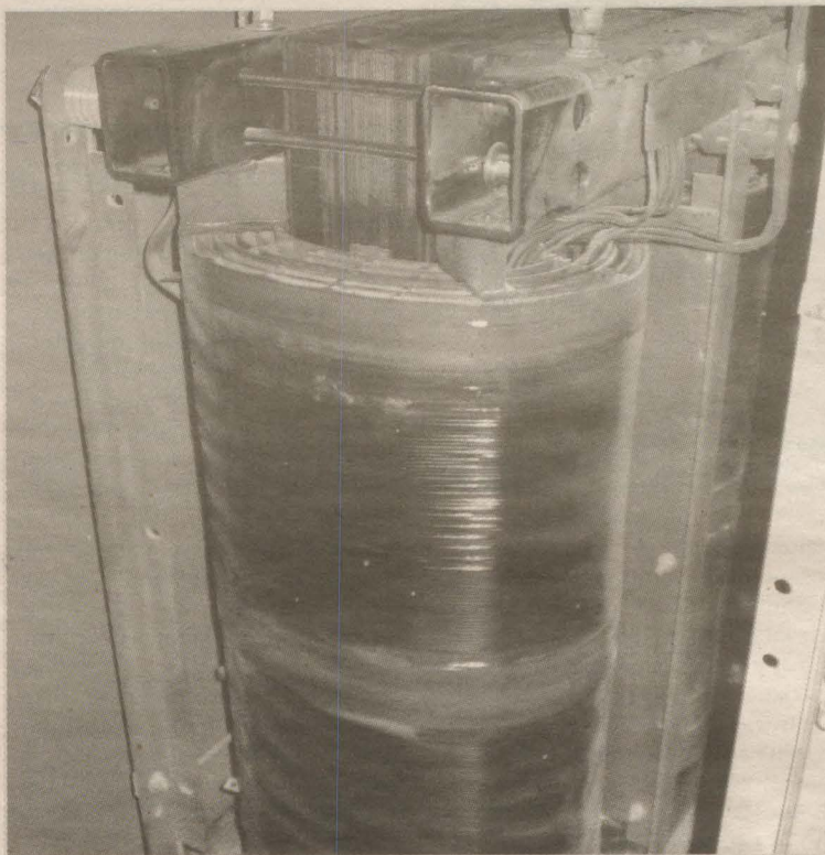
Smoke began to rise in the Killam on March 21 when one of three transformers that power the library suddenly ignited. / Photo courtesy of Facilities Management
