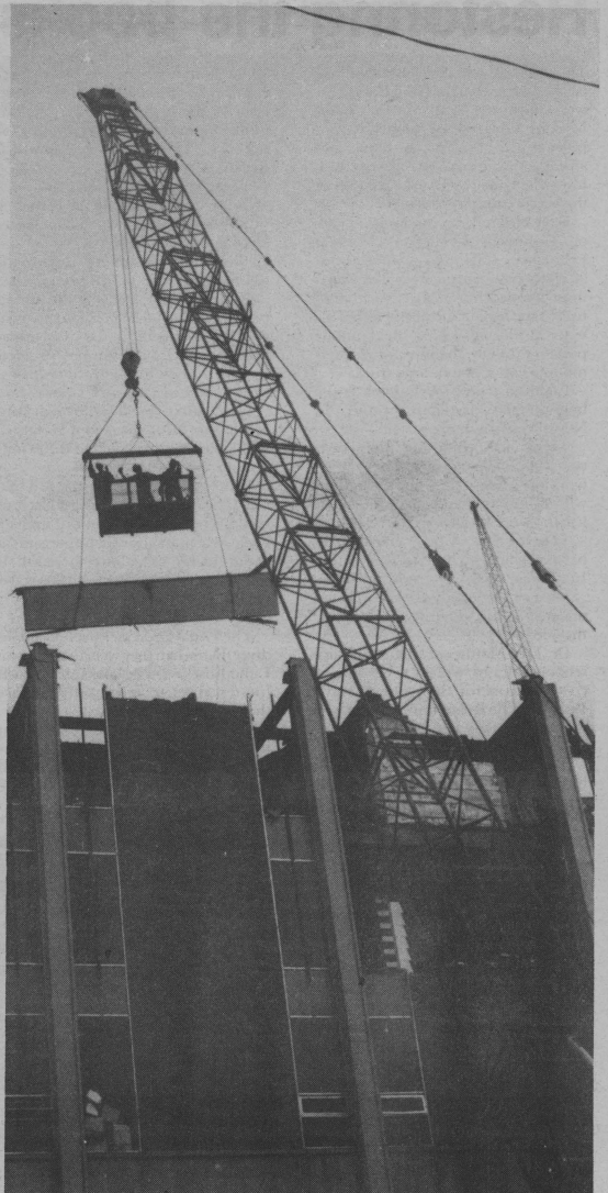
Work crews removed the roof from fire-charred fifth floor on Monday, Aug. 19th. (Watson photo)
