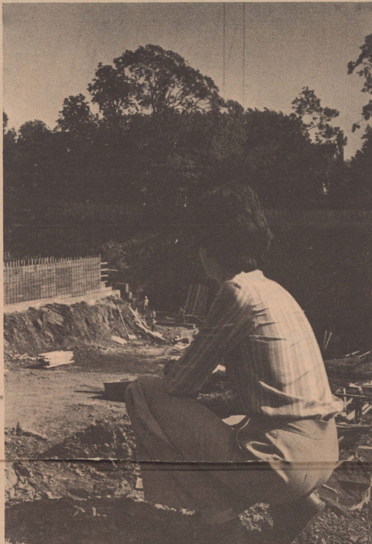
Information Office staffer Kate Carmichael surveys the progress on the Physical Education, Recreation and Athletic Centre, progress that university planner Jim Sykes says is "pulsing ahead" toward the late - 1978 completion target.
