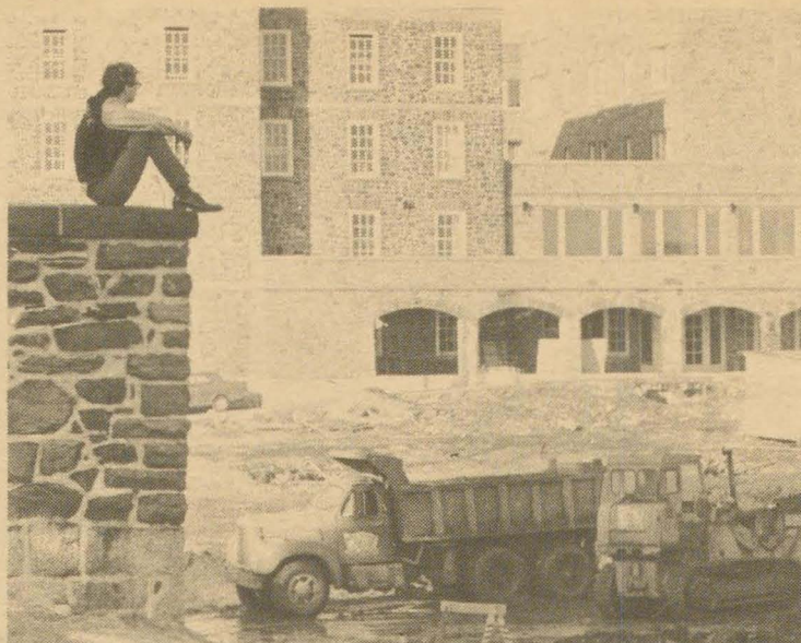
Overnight, a new scar appeared on the face of the campus. The hole currently obstructing traffic in the north-east part of the campus will soon have $6 million poured into it as the five-storey Killam Memorial Library takes shape.
