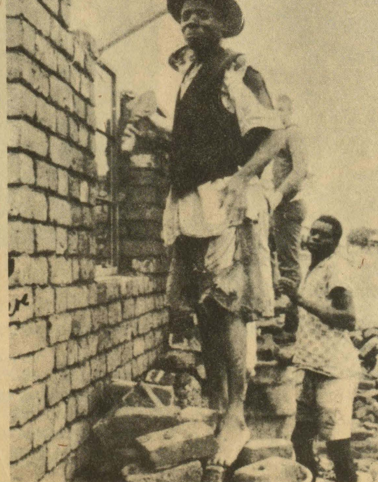
Bill Curry hard at work building a house which is to be part of the St. Francis Hospital complex.
