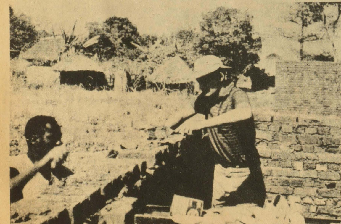
Progress is being made with the bricklaying. The project was in Katete, Zambia. This is one of five houses being constructed.
