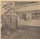
Stainless steel beer cooler with automatic grate control panel in background.
