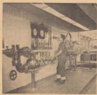
Portion of brewhouse automatic control panel.
