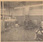
Modern carbonating room showing stainless steel beer lines with pin-point carbonator in background.
