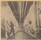
No. 4 storage cifter. Eleven glass lined tanks with a capacity of 15,000 gallons each.
