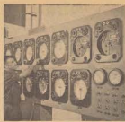
Fermenting foam automatic temperature controls.
