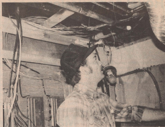
Charlie Beaver repairs damage caused by the fire Sunday morning in the Henson College library. (Watson photo)
