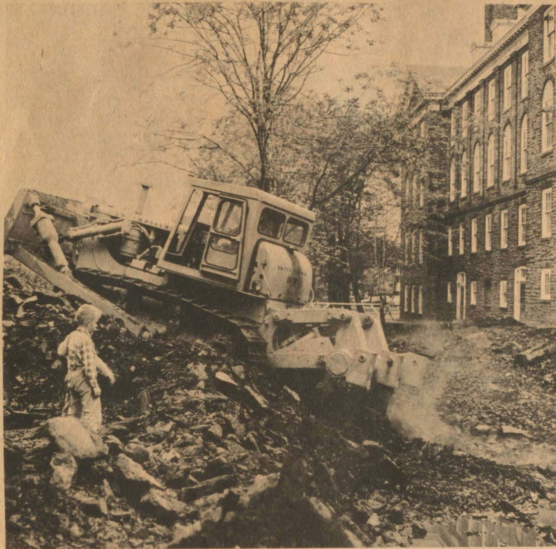
The SUB comes closer as projects are undertaken by construction crews on Dalhousie campus. The New Men's Residence addition is completed, the Chem Bldg. is just started. That leaves as suspected priorities the Law Bldg. and the New Med Bldg.
