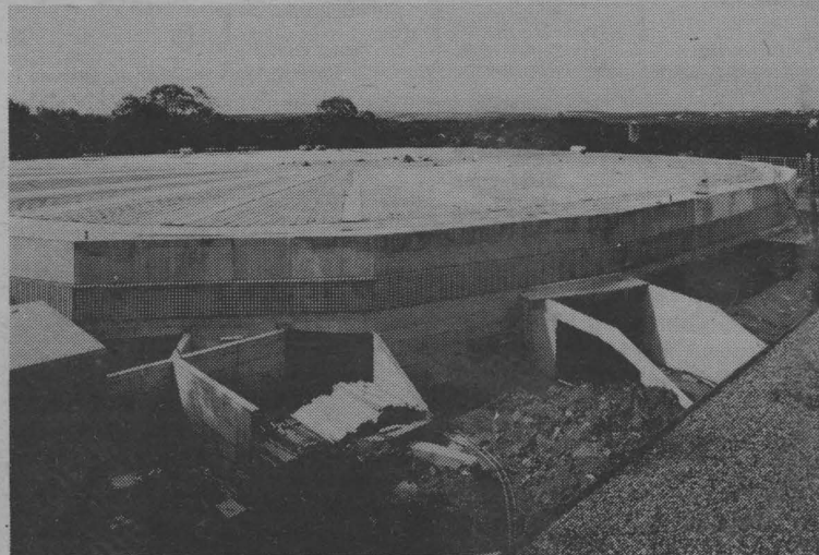
They'll raise the roof of DALPLEX soon. The spring sections for the air-supported stainless steel bubble are already in place. (A/V Services)
