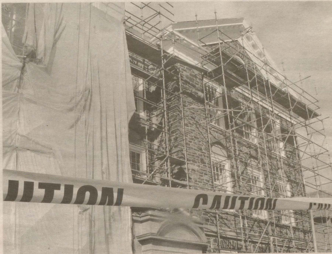
Dalhousie has earmarked roughly $600,000 to restore the Chemistry Building as part of a broader effort to invest in maintenance projects on campus. / Photo: John Packman
