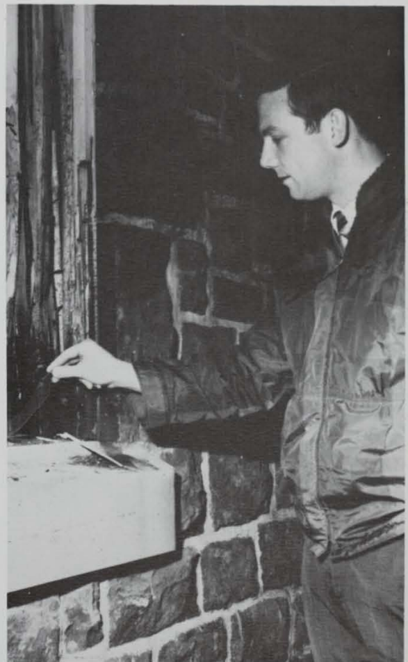
Student Council member, Neil Sharphen examines bomb blast damage.
