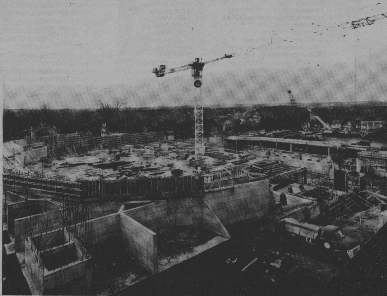
Construction on the new Physical Education, Recreation and Athletic Centre is moving right along—with the roof beams in place, the whole complex is beginning to take shape. The upper platform surface in the picture above is the beginning of the inside track, the Olympic size swimming pool is located on the level under the track.
